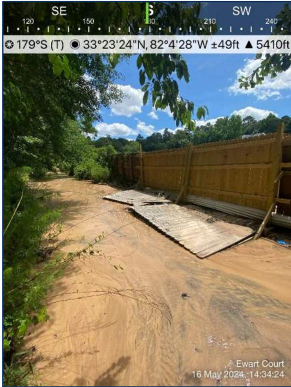
Photograph 1: 2010 Ewart Court, looking upstream at the left bank adjacent to the failing fence line.
