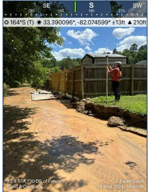
Photograph 4: 2010 Ewart Court, looking upstream at the left bank, just downstream of the failing fence line.
