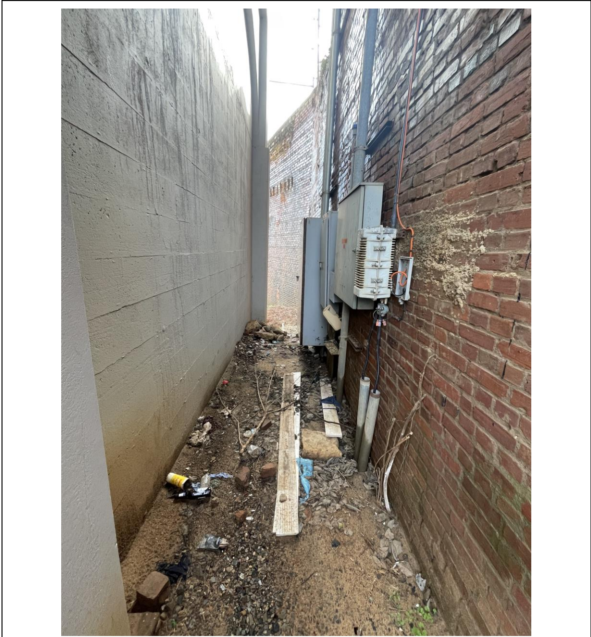
Figure 18. Example where panels need to be secured from public access.
