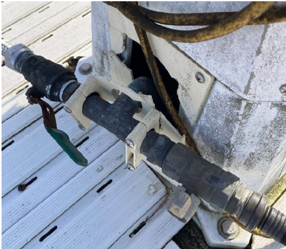
Photo 25 - Typical cracked hose bib on pedestal
