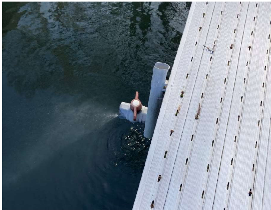
Photo 27 - Leaking water valve near slip 68
