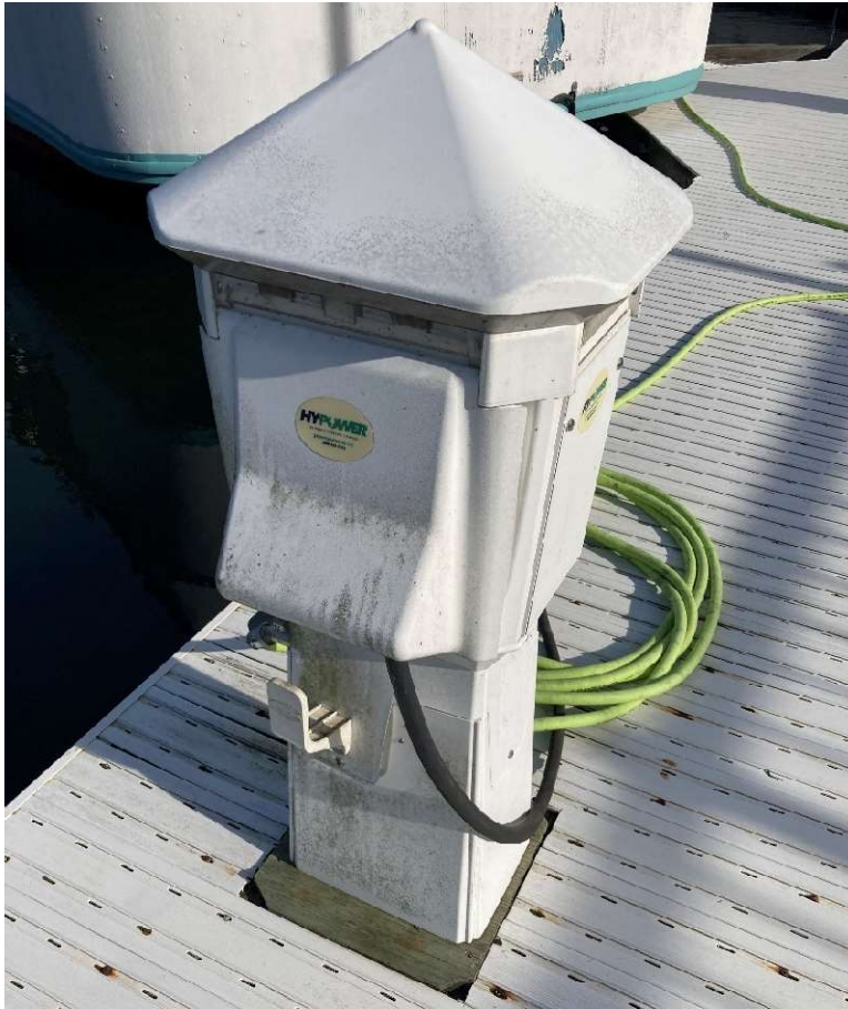
Photo 28 - Typical HyPower brand pedestal
