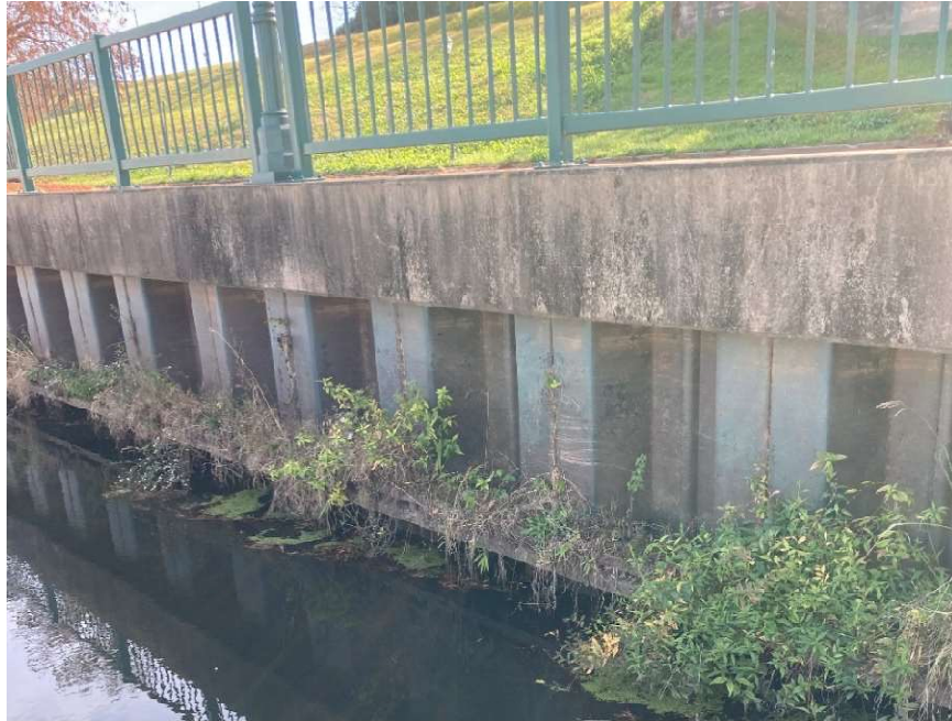
Photo 34 - Vegetation growth on steel waler beam
