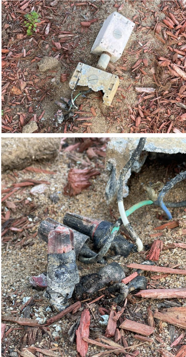
Figure 13. Example of a damaged electrical box with wires that melted/caught fire.
