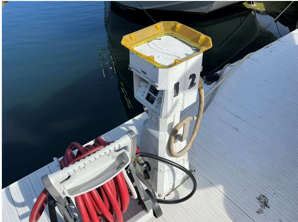
Photo 20 - Missing pedestal top at slips 1/2
