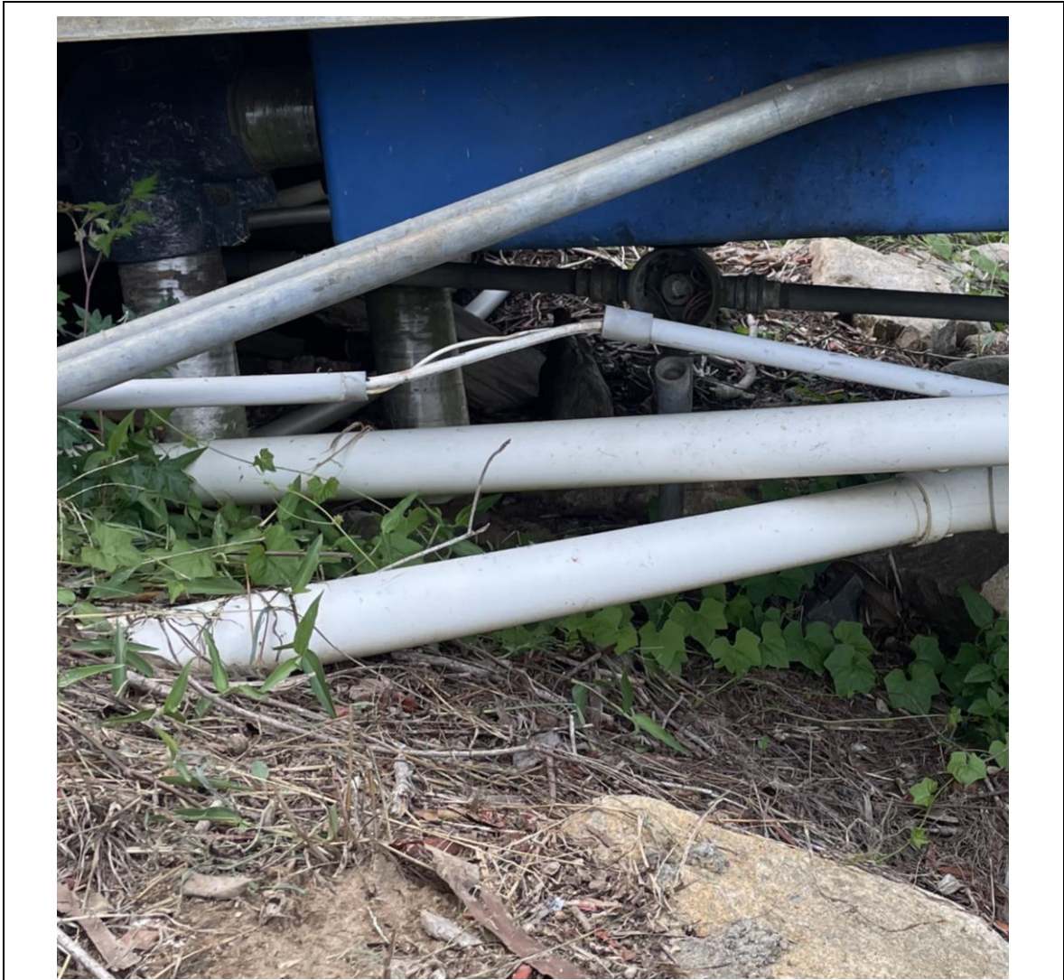
Figure 2. Example of broken conduit and exposed wires.
