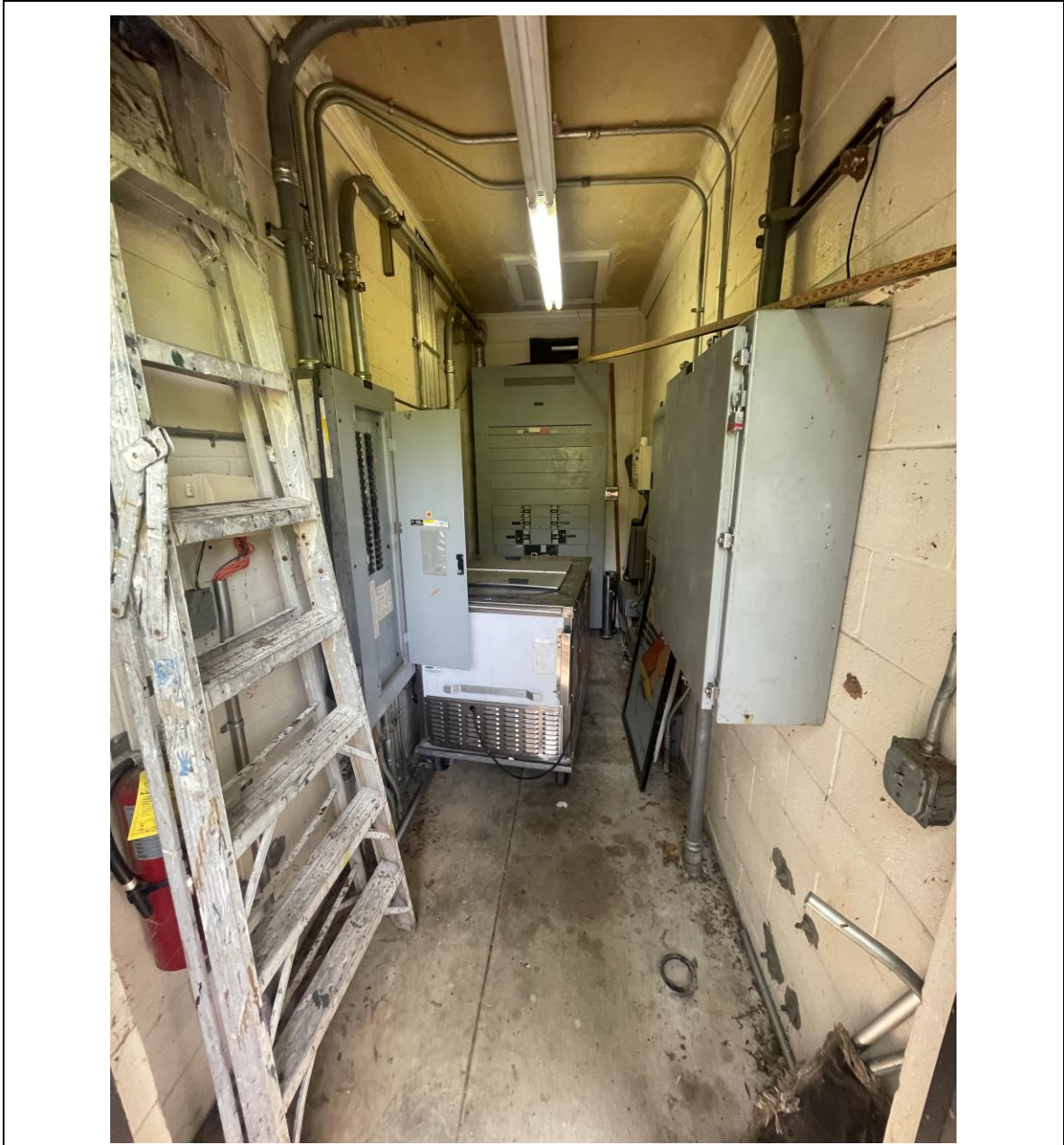
Figure 17. Example where 2020 NEC working space clearances need to be marked.
