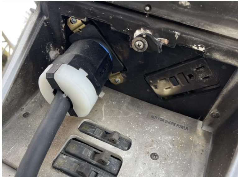
Figure 9. Example of an electrical fire on a shore power pedestal.
