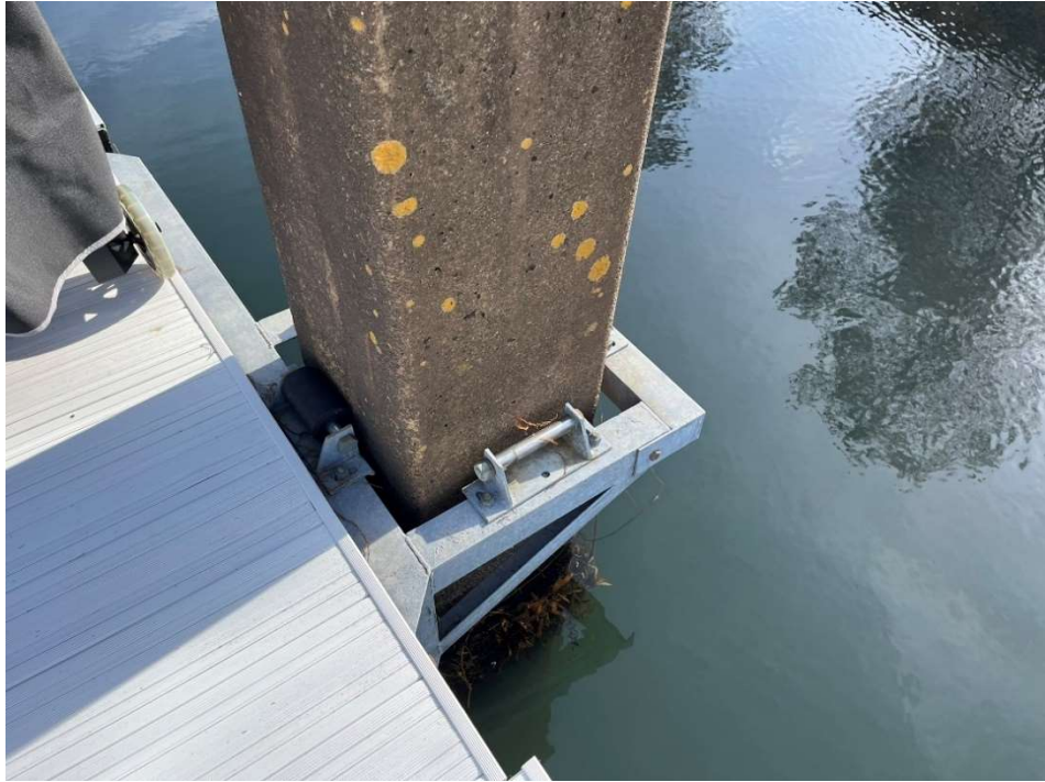
Photo 7 - Missing HDPE roller on pile guide
