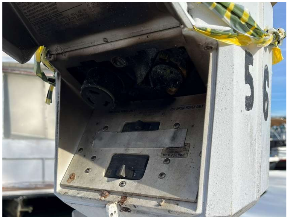
Photo 21 - Burn marks on slip 5/6 pedestal that reported caught on fire
