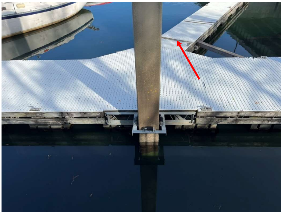
Photo 6 - Typical concrete anchor pile (note missing vinyl decking)
