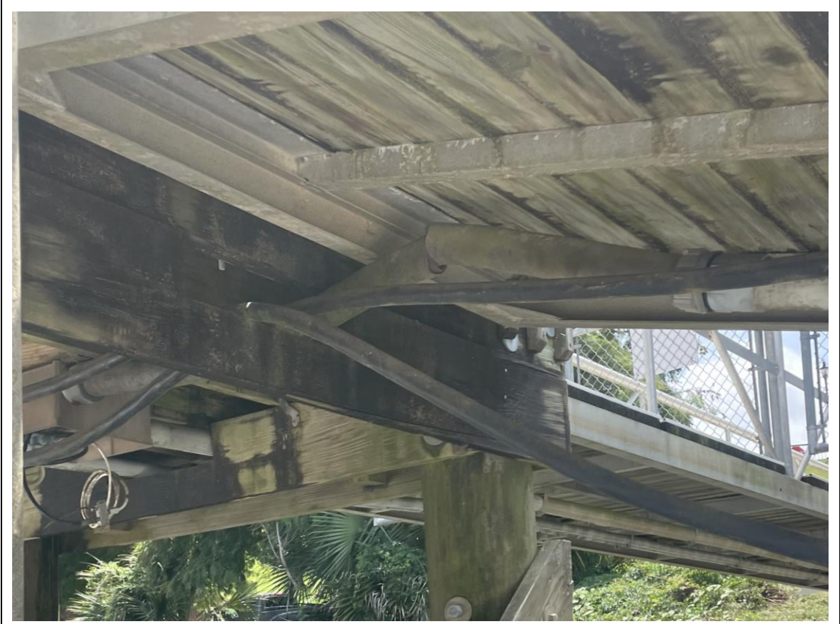
Figure 4. Example of broken conduit.
