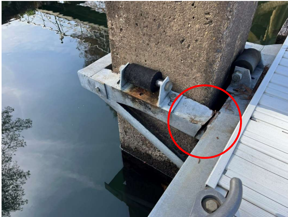
Photo 5 - Broken pile guide near slip 11/12
