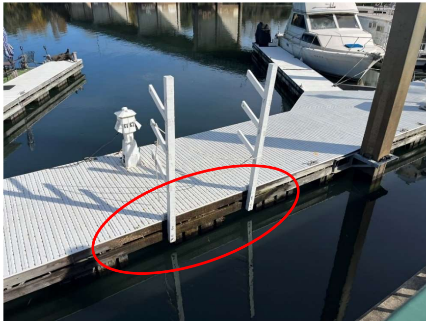
Photo 13 - Water leak near slips 61/62
