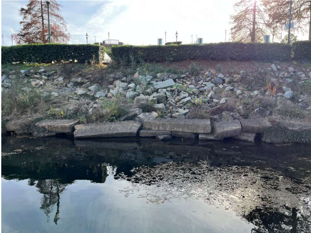
Photo 32 - Apparent settling angular stone & toe stone
