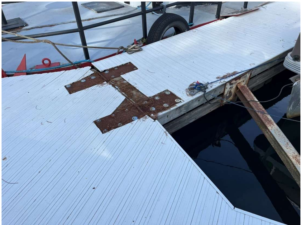
Photo 4 - Large steel bracket near slips 9/10
