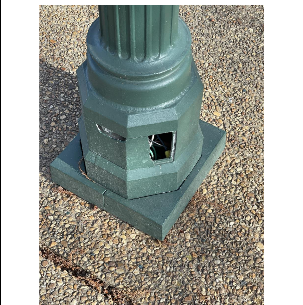
Figure 12. Example of a damaged light pole base that has exposed wiring.
