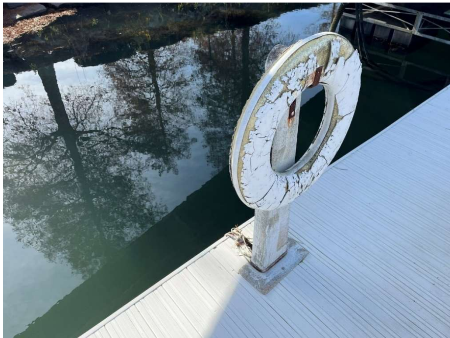
Photo 23 - Severely deteriorated life ring
