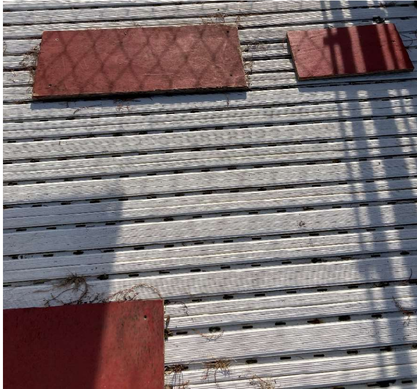
Photo 19 - Plywood patches on B-2 Access Platform
