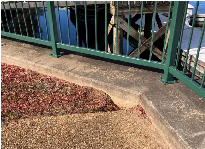
Photo 35 - Minor backfill loss observed near B-1 access location
