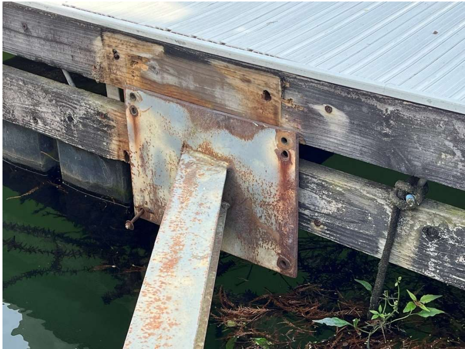
Photo 3 - Detached supplemental angle bracing near slip 10
