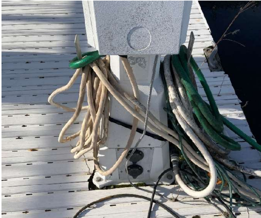
Photo 26 - Numerous spliced power cords at slips 43/44
