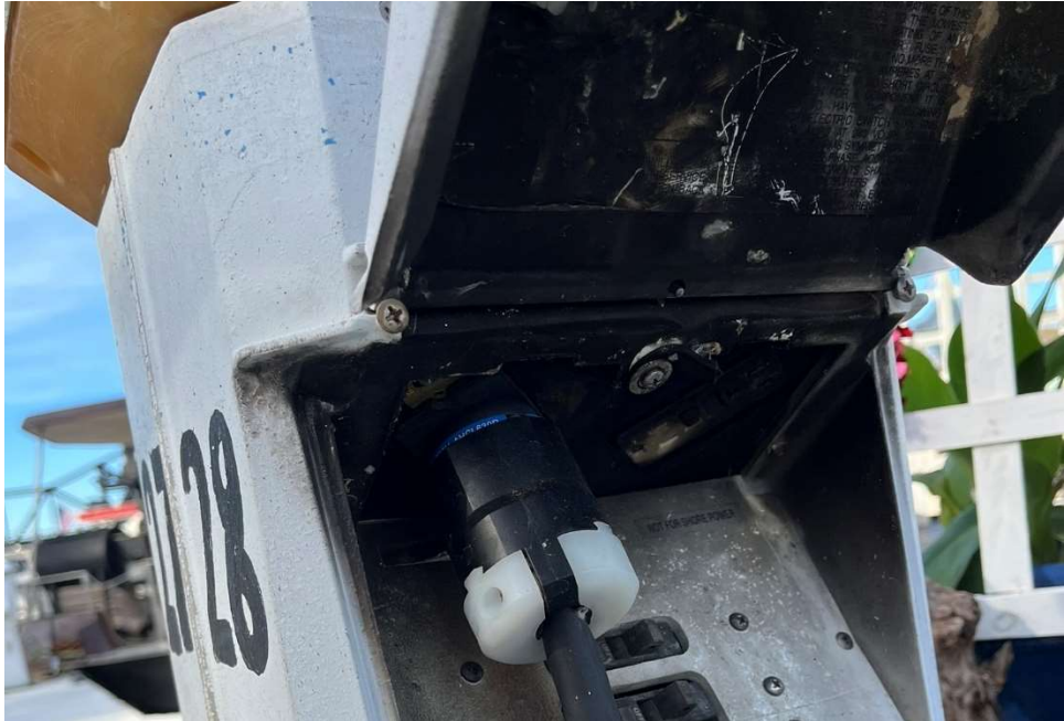
Photo 24 - severely charred pedestal receptacle at slips 27/28
