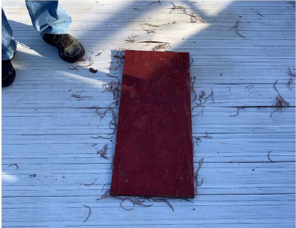
Photo 1 - Plywood patch on decking near service dock area
