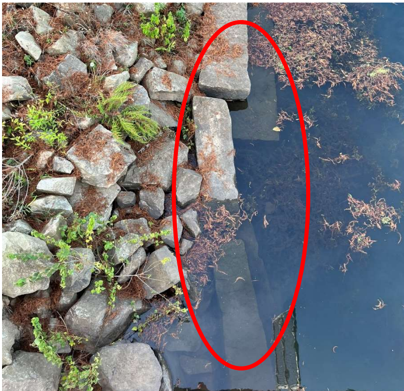
Photo 31 - Apparent settlement of toe stones
