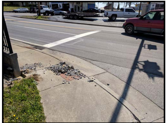
Main St. and Stratton/Elizabeth Deficient DWS, Ramp with no Crosswalk
