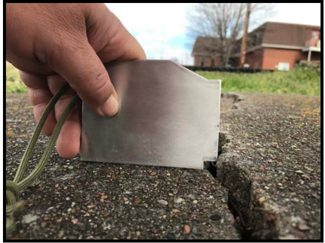
HWY 49/Frey Street- Typical Discontinuity >1/4"
