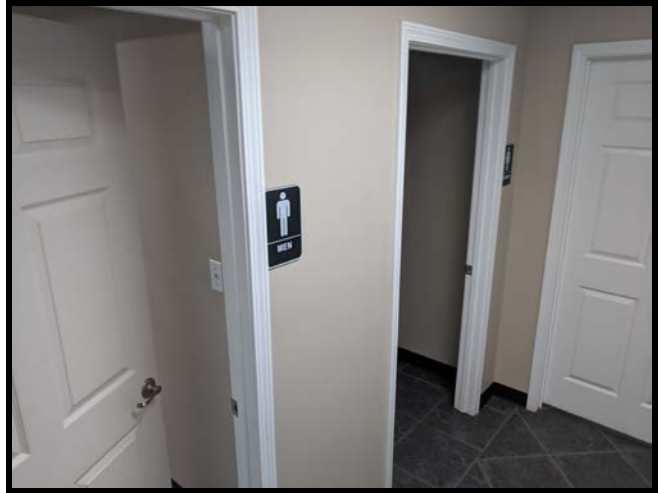
Parks/PW Dept. Restroom, Non-Compliant Signage
