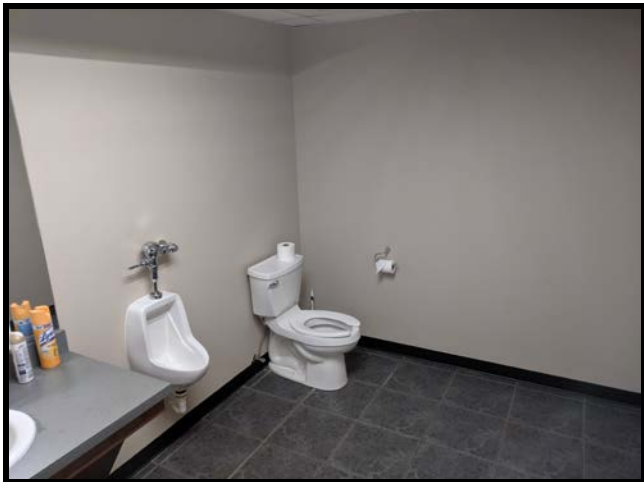
Parks/PW Dept. Restrooms, No Safety Handle
