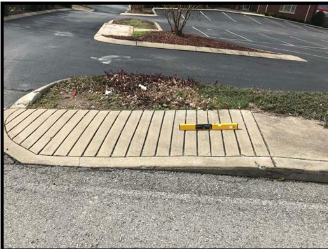
Duke Street- Running Slope of Ramp >8.3%
