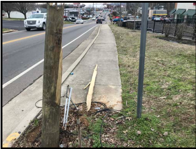
Main Street/HWY 12 Utility Pole Obstruction and No Clear Path
