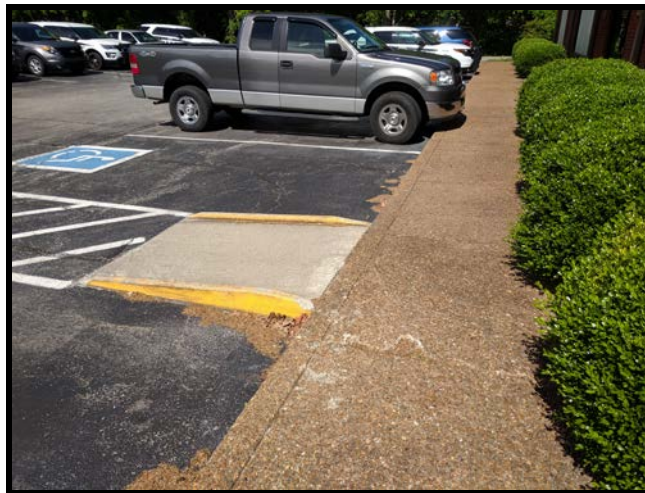
Police, Parks & PW Ramp and Sidewalk Deficiencies
