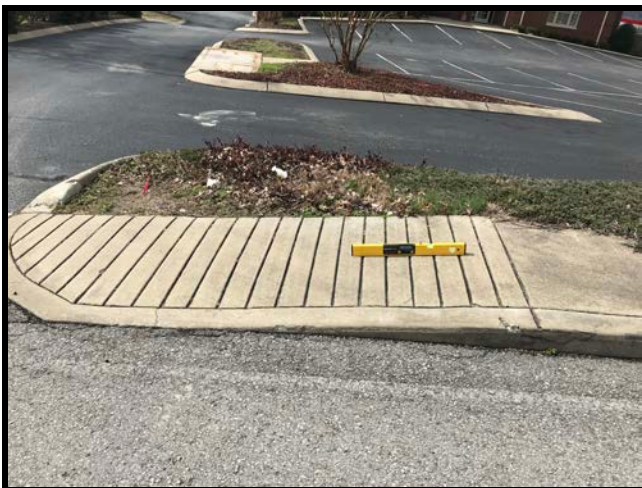
Duke Street- Running Slope of Ramp >8.3%
