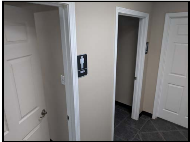
Parks/PW Dept. Restroom, Non-Compliant Signage
