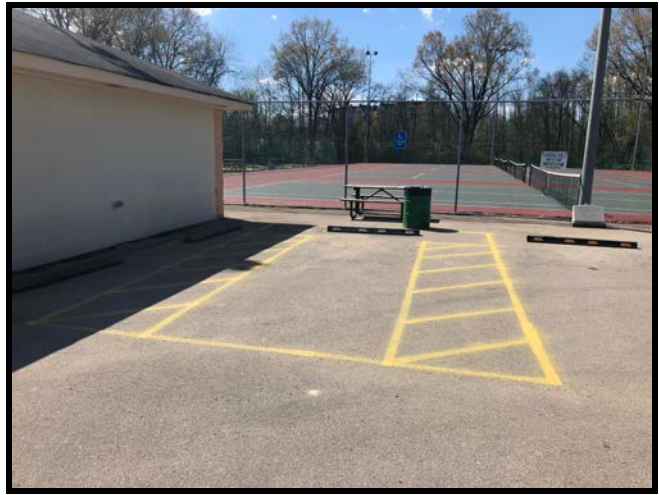
John C. Poole Parking Space & Aisle Non-Compliant
