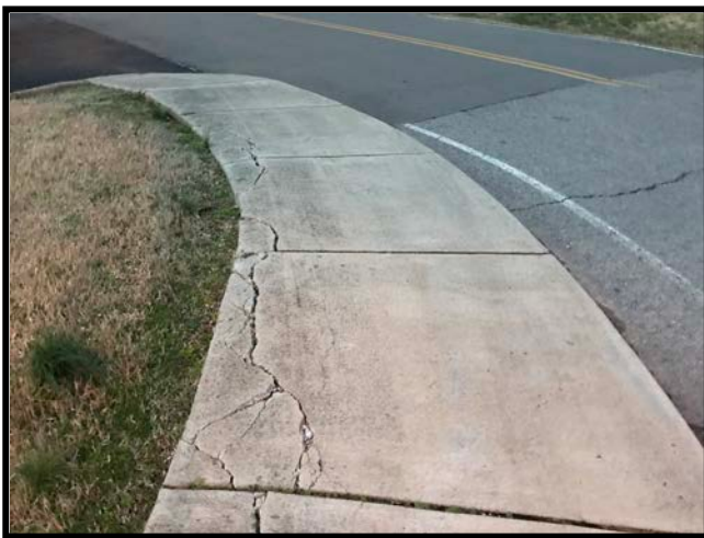
Ruth Street- Cracked Sidewalk and Cross Slope >2%
