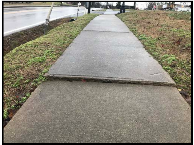
Main Street/HWY 12-Typical Discontinuity >1/4"
