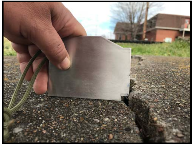
HWY 49/Frey Street- Typical Discontinuity >1/4"
