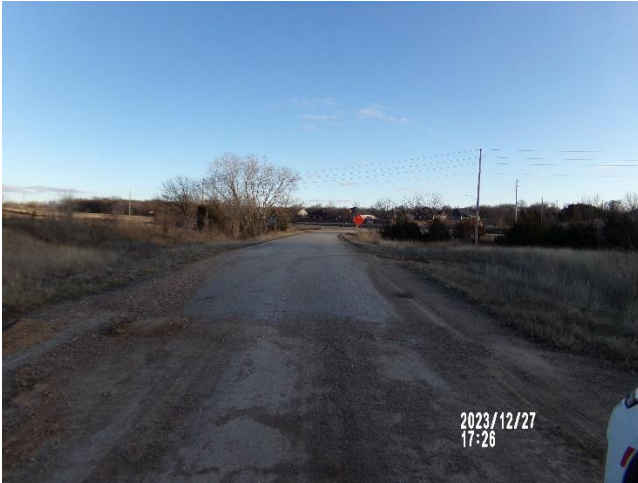
End of pavement approx 400 feet north of intersection, south of site taken 12/27/2023 by Josh White
