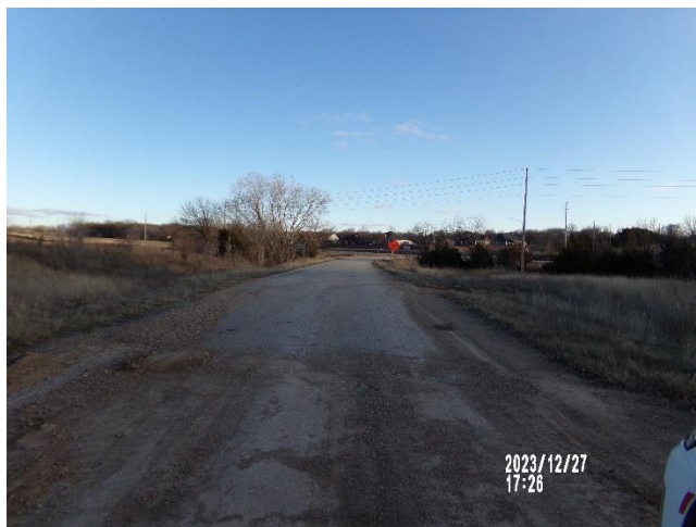
End of pavement approximately 400 feet north of intersection, south of site taken 12/27/2023 by Josh White
