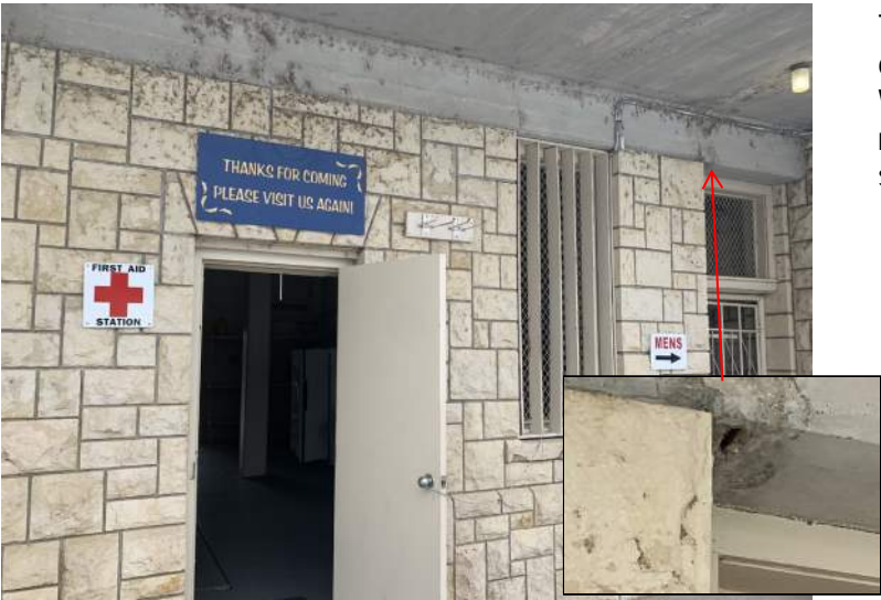
The most severe damage observed in this overhang is shown in the photo inset. Water intrusion has corroded the reinforcement causing the concrete to spall on the bottom of the member.
