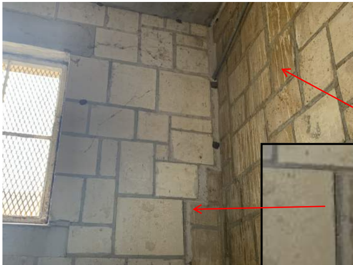
Note a gap has opened up since the tuck point repair indicating continued movement in the structure. This is in the storage room on southwest corner of building.
