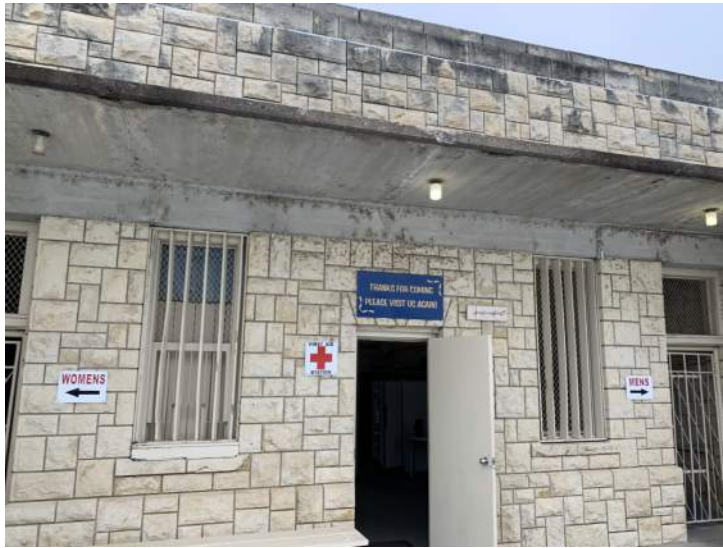
The concrete slab overhang shows cracking and distress most likely from water intrusion due to poor drainage. The dark patches along the the bottom side where the slab meets the wall may indicate mildew and potentially spalling of concrete. The slab exhibits lateral cracks extending through the width of the overhang.
