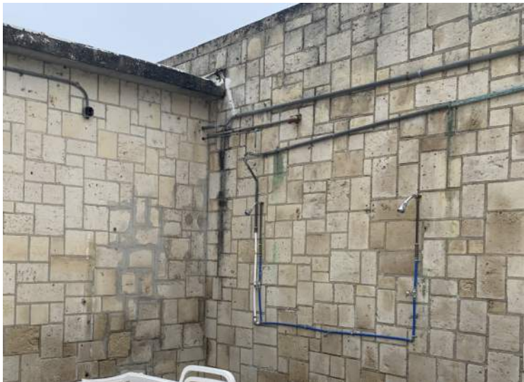
The next two photos show earlier tuck point repairs in the masonry joints to address cracking due to settlement.
