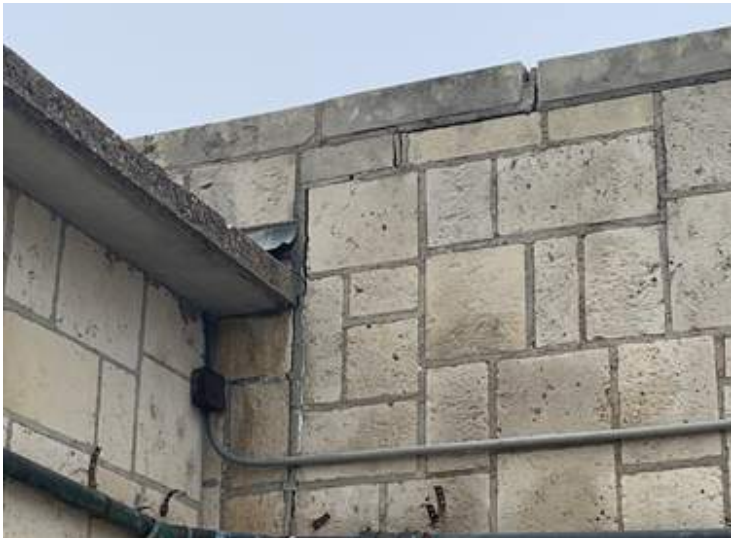
Damage due to settlement in the opposite (northeast) corner of the building from the previous photograph.
