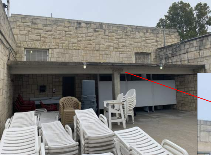
The roof overhang in the men's changing area show deterioration. Note the damage at the top of the center column and the cracking, spalling, and exposed reinforcement along the edge of slab.
