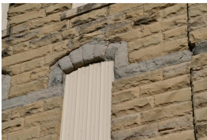
226 S. Summit. 12-12-2017. Detail of cement parging on lintels and beltcourse (typical). B. Spencer
