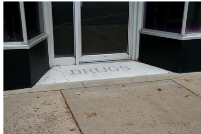
110-114 S. Summit. Cararra glass bulkhead and hex tile at recessed entry at south storefront bay. 11/14/2017. B. Spencer
