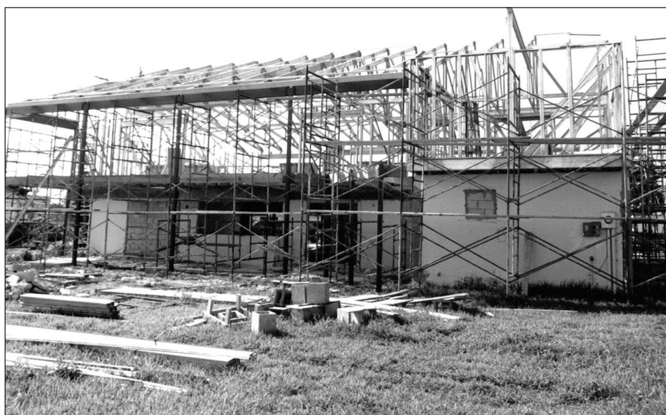
Figure 3-12. The owner of this flood-prone home in south Florida decided to build a new wood-framed second story on top of the masonry first story. The new second story is well above the BFE.
