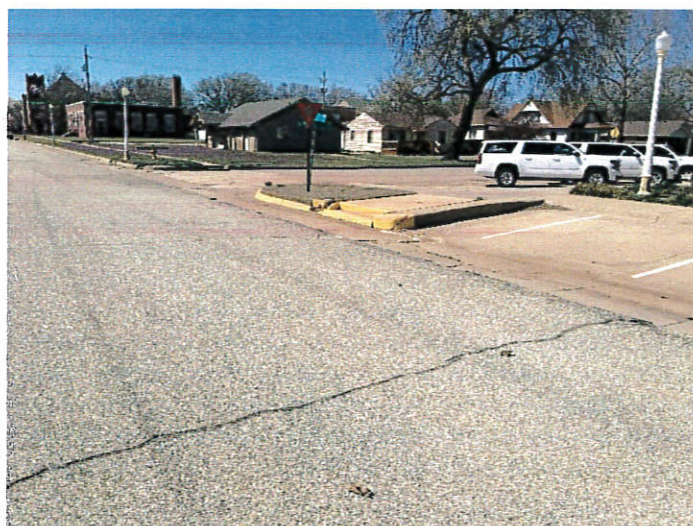
Sidewalk at the corner of Steadman St. and Jennings Ave.
