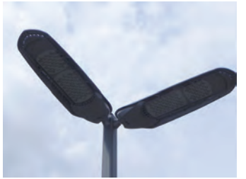
Path lighting along Princess Anne Road corridor
