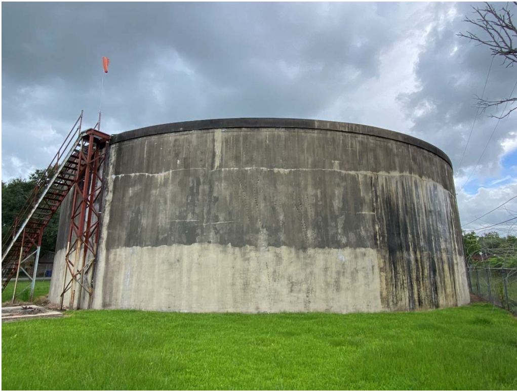
Exterior Wall with Horizontal Crack and Leak
