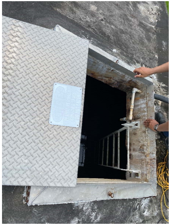
Dome Vent and Access Hatch
