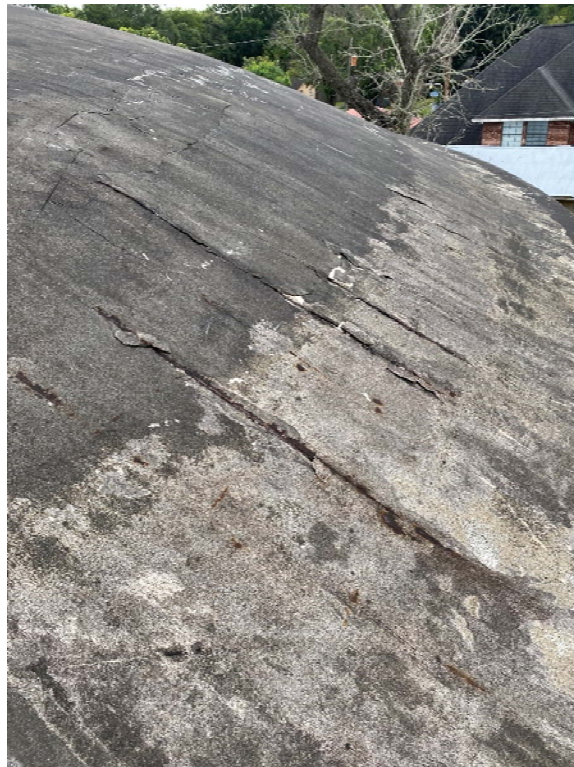
Exterior Dome Surface with Cracking and Exposed Reinforcing
