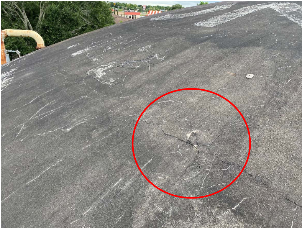
Overall View of Dome. Note cracking in foreground.
