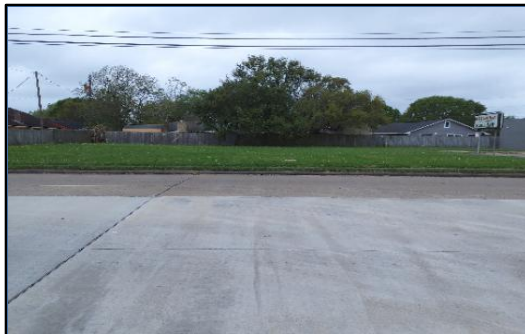
Corner 4 No Ramp (4z)
