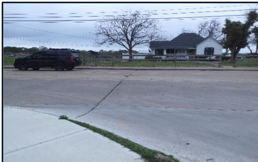
Corner 4 No Ramp (4z)
