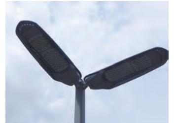
Path lighting along Princess Anne Road corridor
