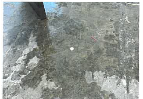
Lobby; area flooded
