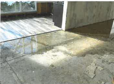
Lobby; area flooded
