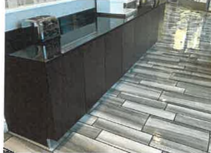
Lobby; affected area
