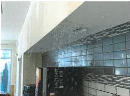
Lobby; affected area
