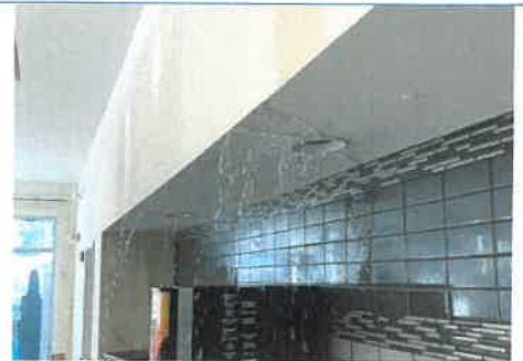
Lobby; water coming through ceiling and lights
