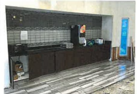
Lobby; affected area
