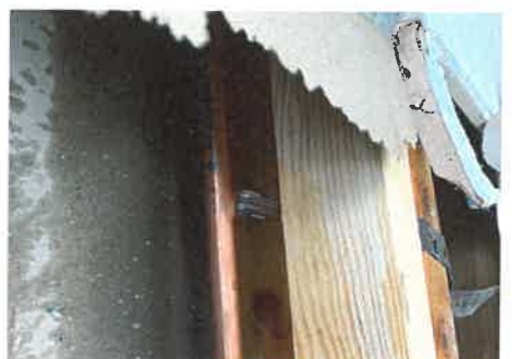
Lobby; pipe break
