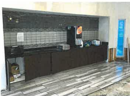
Lobby; affected area
