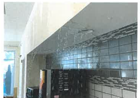
Lobby; affected area
