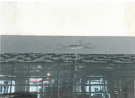
Lobby; affected area
