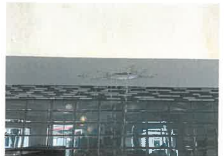
Lobby; affected area
