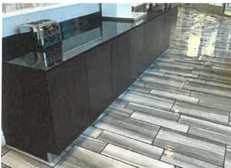
Lobby; affected area
