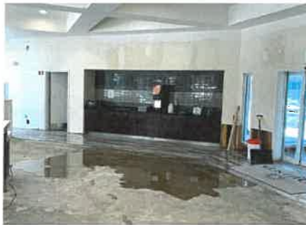
Lobby; affected area
