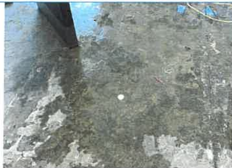
Lobby; area flooded
