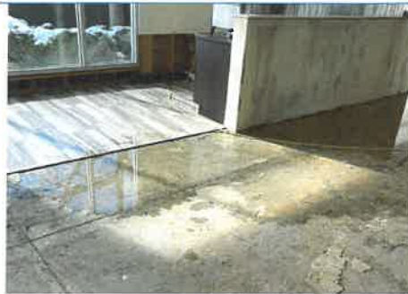
Lobby; area flooded
