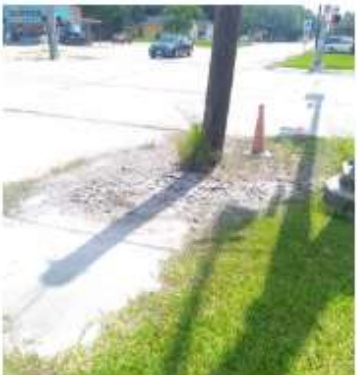
Existing Cracked Sidewalk and Poor ADA Facilities
