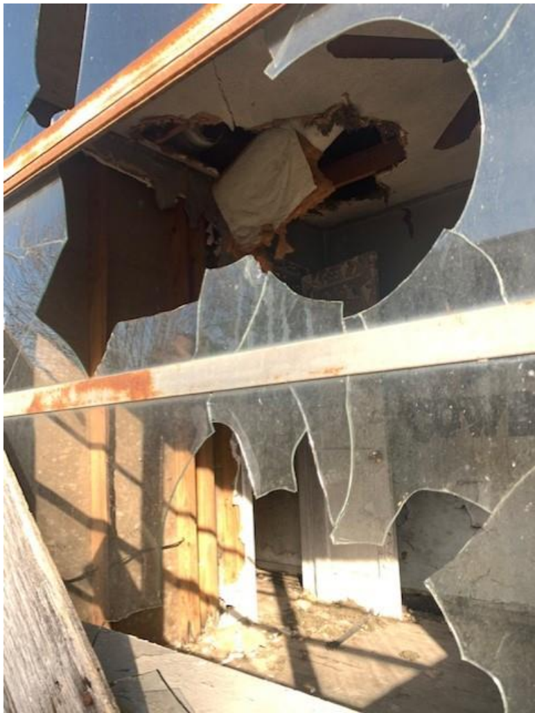
Broken windows, ceiling caved in
