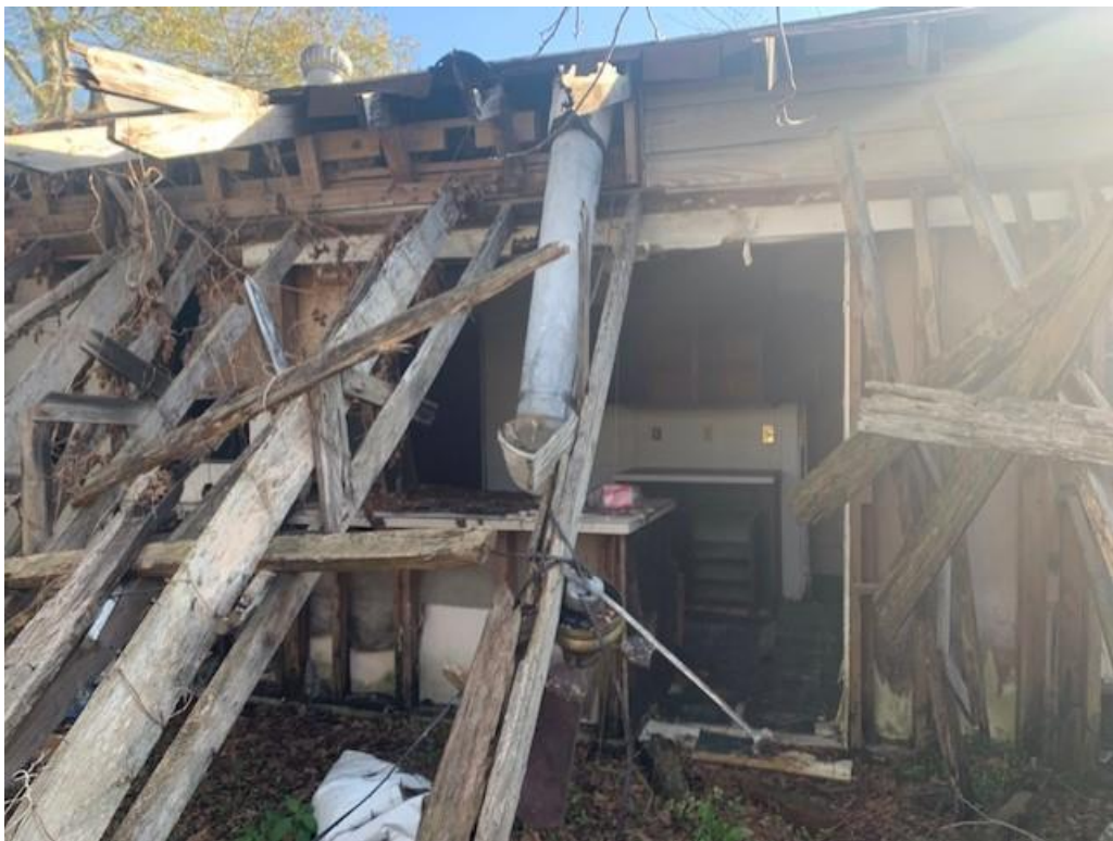
Kitchen visible - back wall missing
